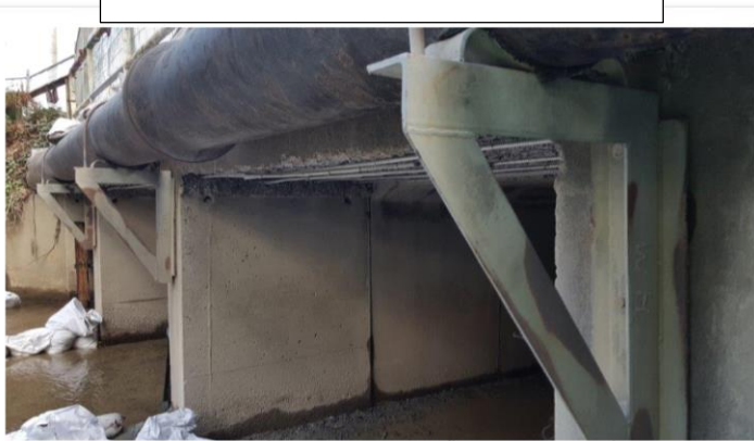
Temporary propping before Andersal Pty Ltd works commenced because council was concerned a vehicle mounting the kerb would cause the failure of the footpath.
