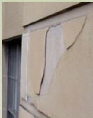
WHEN SPRING CALLS, BUILDING SPALLS AND ITS "FOLIAGE" FALLS
