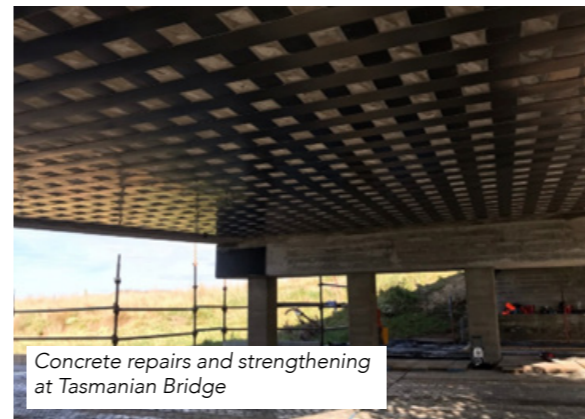
Pensar restored and strengthened a number of ageing concrete bridges in regional Tasmania
