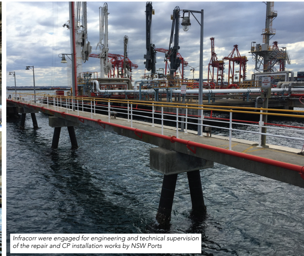
Extending the service life of the wharf structure at the Bulk Liquids Berth No 1 (BLB 1) Terminal, Port Botany
