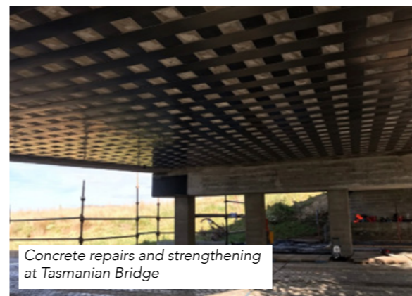
Pensar restored and strengthened a number of ageing concrete bridges in regional Tasmania
