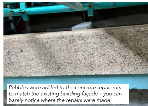
This is a large-scale repair to rebuild the concrete wall structure to match the original profile
