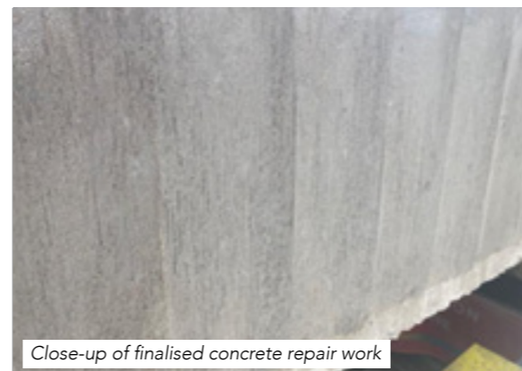
Pebbles were added to the concrete repair mix to match the existing building façade – you can barely notice where the repairs were made
